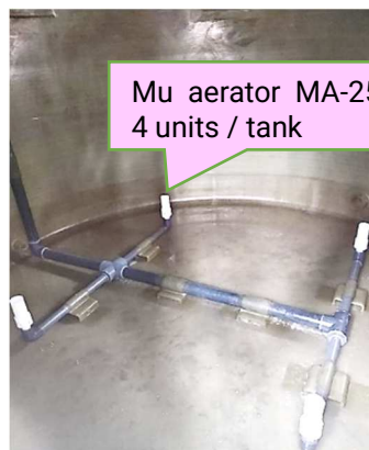
Photo-2 Stirring water tank using a Mu-Aerator
